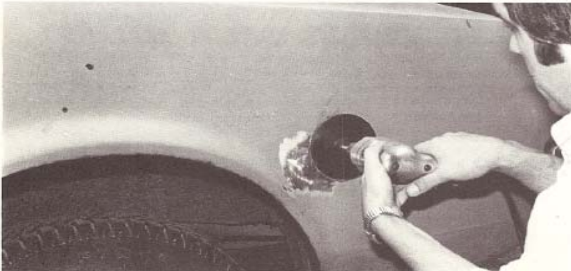
Step 2. Using an 80-grit grinding disc on an electric drill grind the paint from the surrounding area down to bare metal. This will provide a rough surface for the body filler to grab
